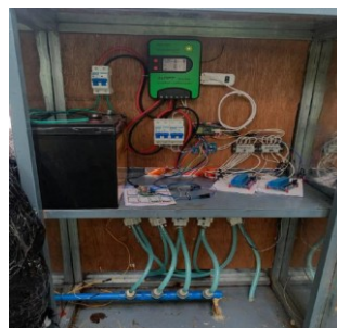
Figure 5. Control unit and sensor integration during operational testing
